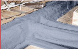
HVAC SYSTEM INSULATION
